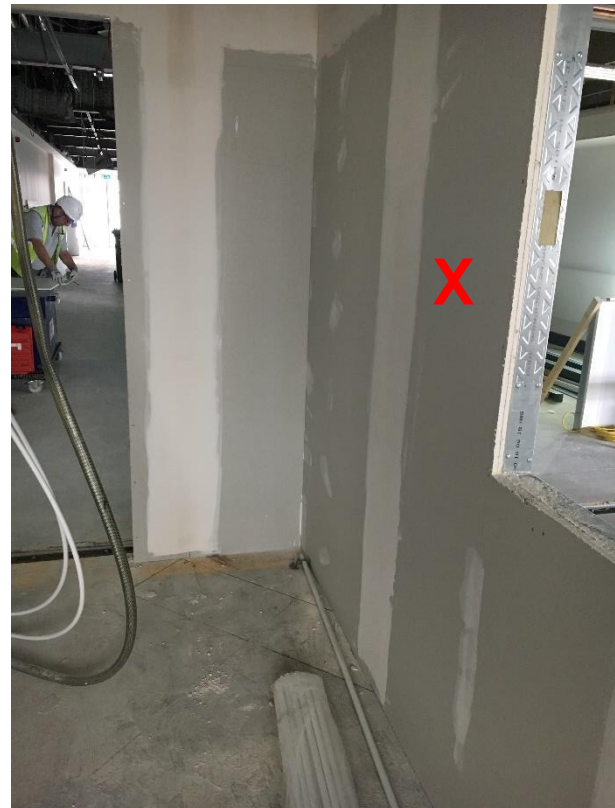
Proposed location of the electronics chassis. Needs to be at a serviceable height accessible from the floor.
